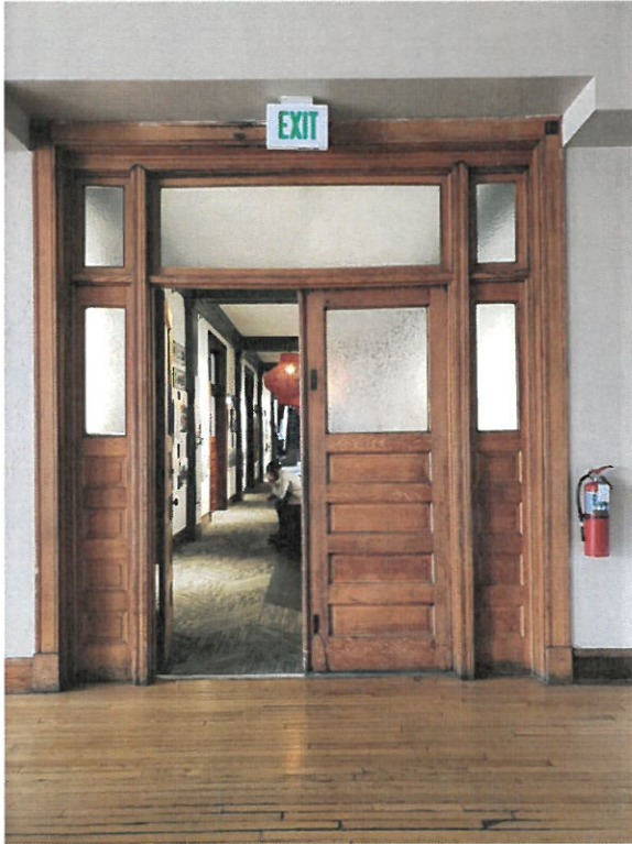
Fire extinguisher; North wall inside Auditorium
