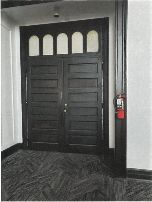
Fire extinguisher; Second floor, outside west theatre door
