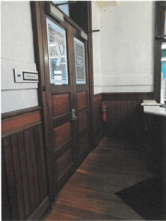
Fire extinguisher; First floor, between entrance to Play & Learn and YMCA main desk
