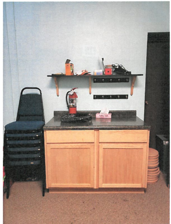
Fire extinguisher; Second floor, room between Ambry and preschool (YMCA)
