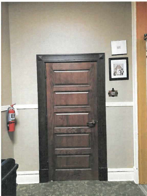
Fire extinguisher; Second floor, Trina's office
