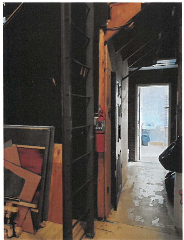
Fire extinguisher; Theatre, rear stage right
