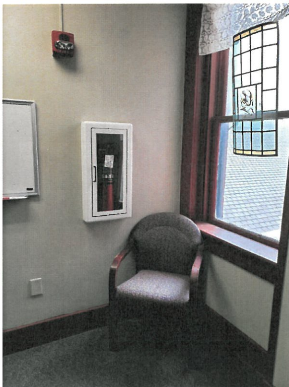
Fire extinguisher; Third floor, southeast corner of hallway in Athenaeum Foundation office
