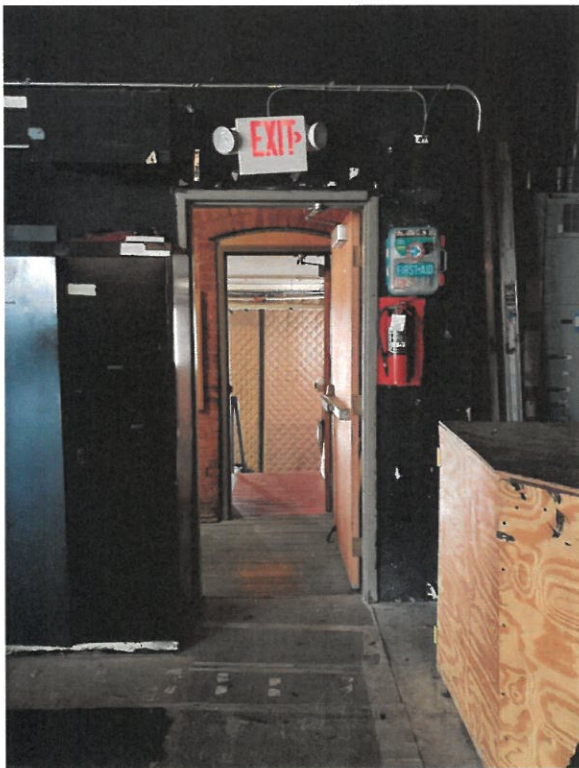
Fire extinguisher; Theatre, rear stage left
