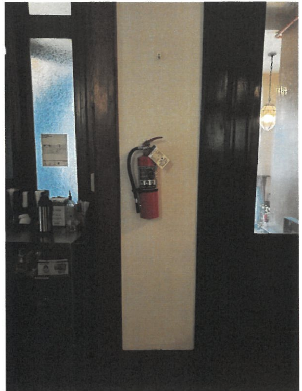
Fire extinguisher; First floor, north wall across from Coat Check Coffee
