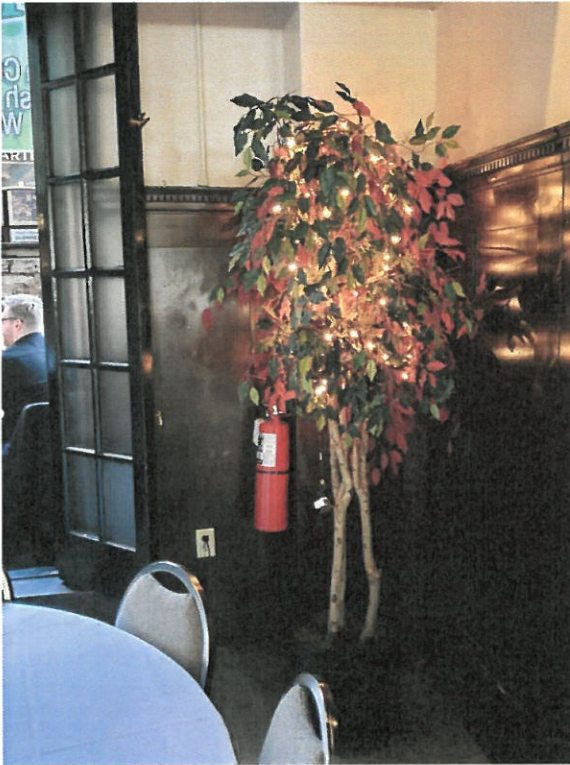
Fire extinguisher; Basement level, east wall in the Grand Kellersal
