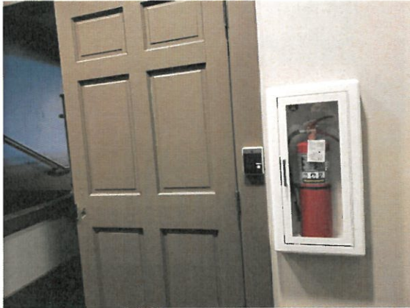
Fire extinguisher; Third floor, inside elevator vestibule
