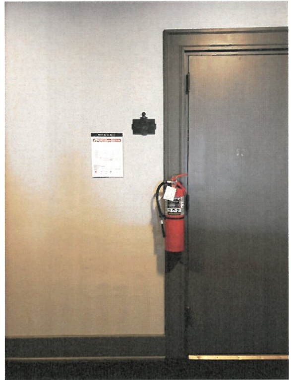
Fire extinguisher; Third floor outside Athenaeum Foundation office
